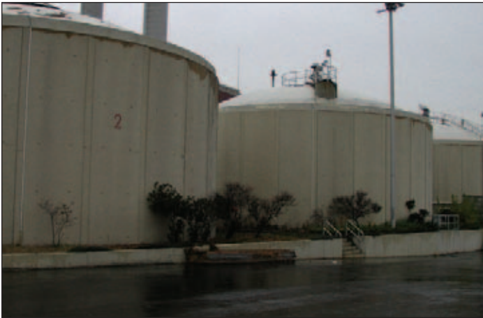
Digester sludge is stored temporarily in a sludge storage tank prior to dewatering and while awaiting shipment to a plant with a dewatering facility
