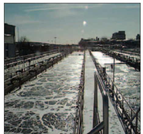
View of Centrate Tank at 26th Ward WPCP
